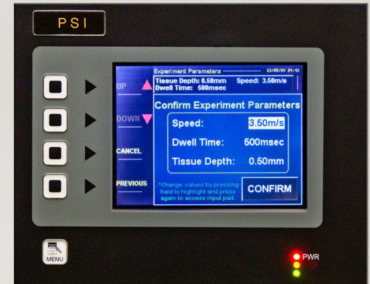
Control Panel Detail
